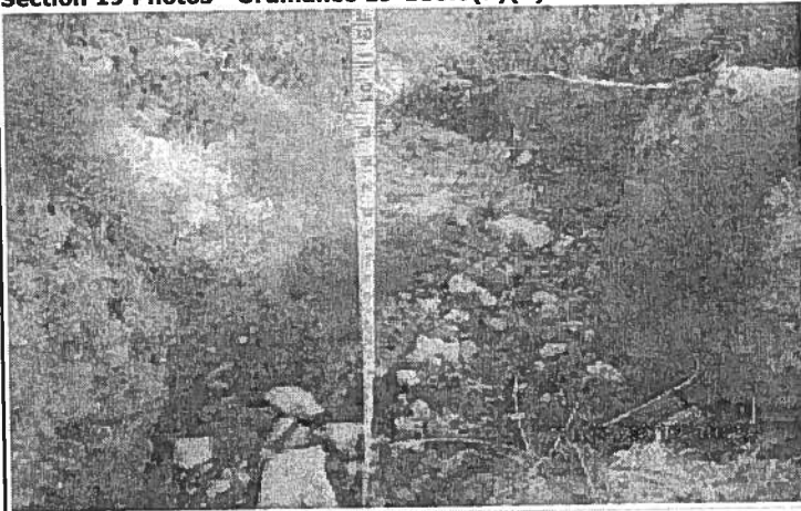
A different erosion gulley 5 ft deep on-site, this is on the south portion of the site.
