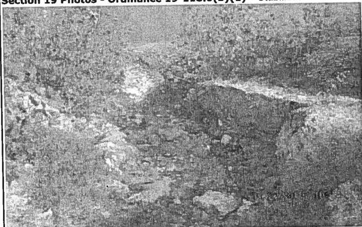
Inside one of the sloughed caved-in gulleys on-site.
